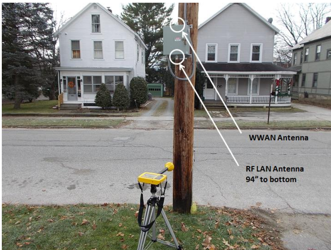
Figure 37. GMP Gatekeeper mounted on a power pole at GMP site 8 with the WWAN antenna on the top and the 900 MHz RF LAN antenna on the bottom.
