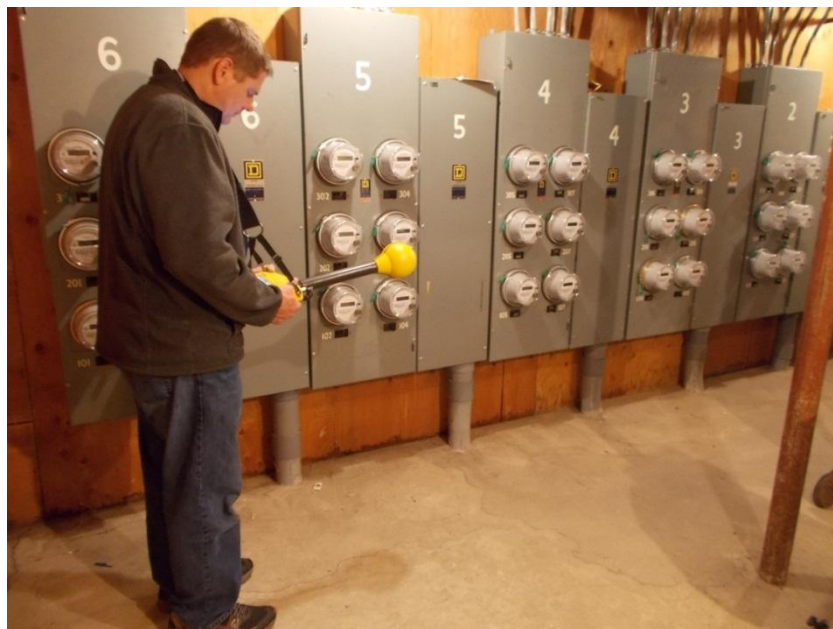
Figure 21. BED site 10 with 36 smart meters inside an electrical room.
